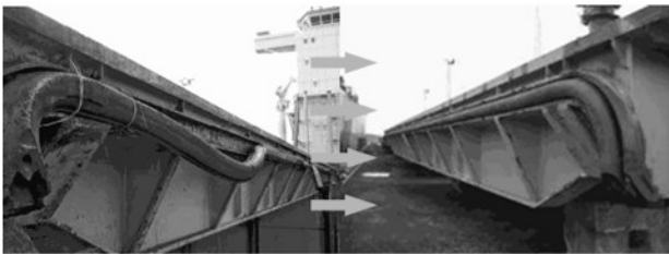
Damaged EVA- Seal Replaced by Deumareco Sliding Seal.
